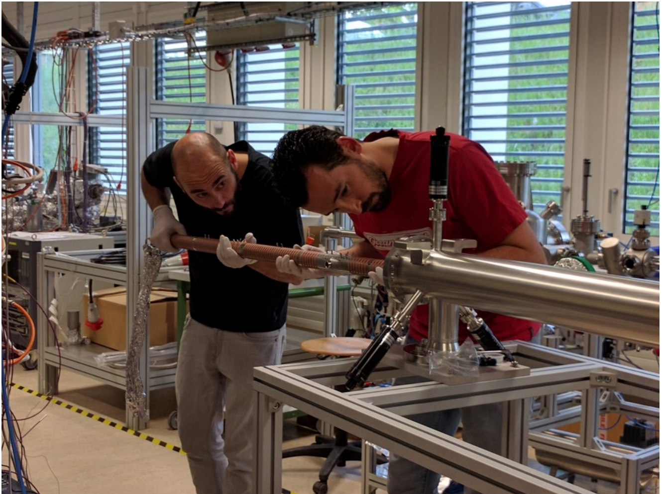
Fig.2: Left Luis Antonio González, Right Left Miguel Gil-Costa during installation of the first FCC-hh beam screen prototype for commissioning at BESTEX. (Image: FCC)
